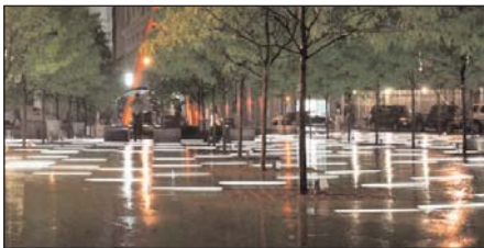
B-K Lighting designed and manufactured custom fixtures for Liberty Park Project in New York City.
